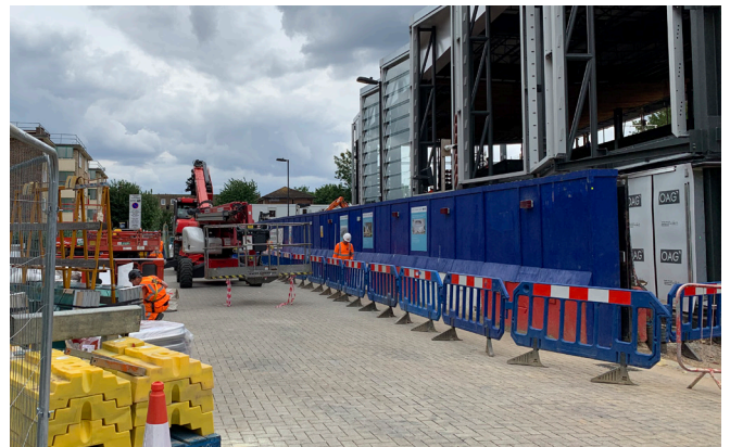
The CBPP paved highway withstood heavy construction traffic during the new station construction.
