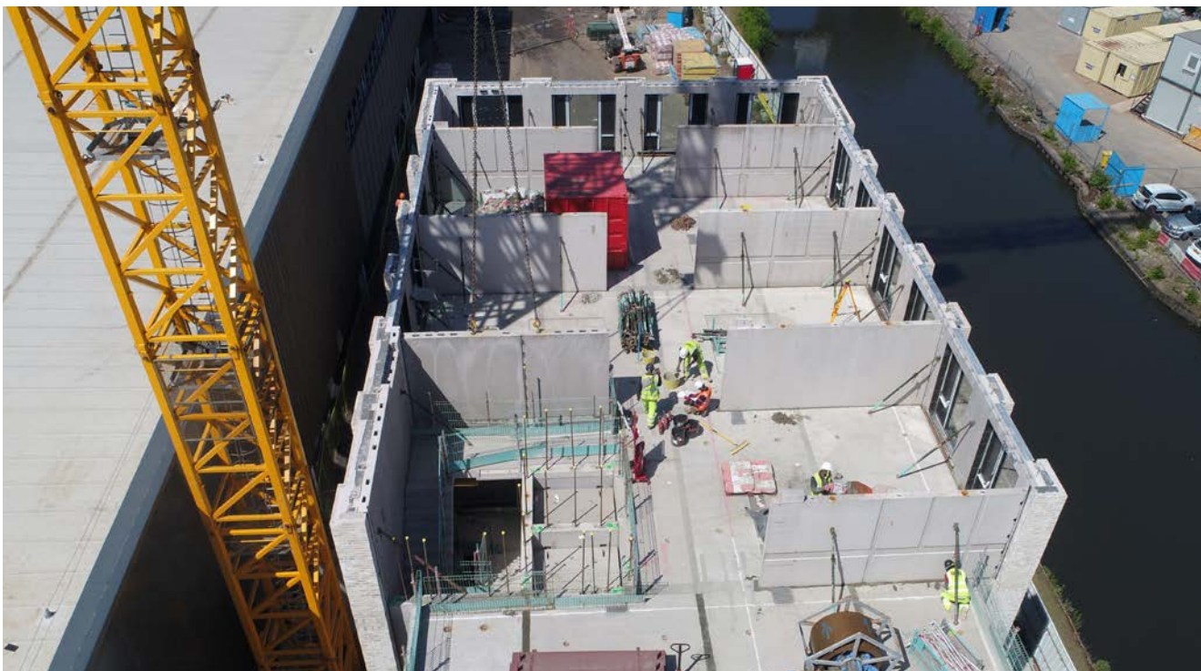
Selly Oak student accommodation, Birmingham. The client has future proofed the building by leaving out every other solid wall so that it could potentially be changed from student accommodation to residential in the future by removing these walls. Image courtesy of FP McCann.
