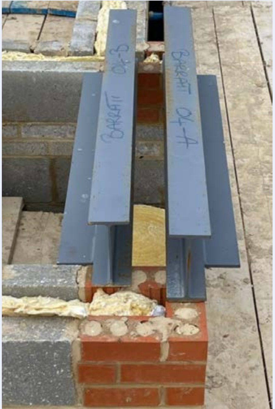
Figure 3 Example of unstable beam
