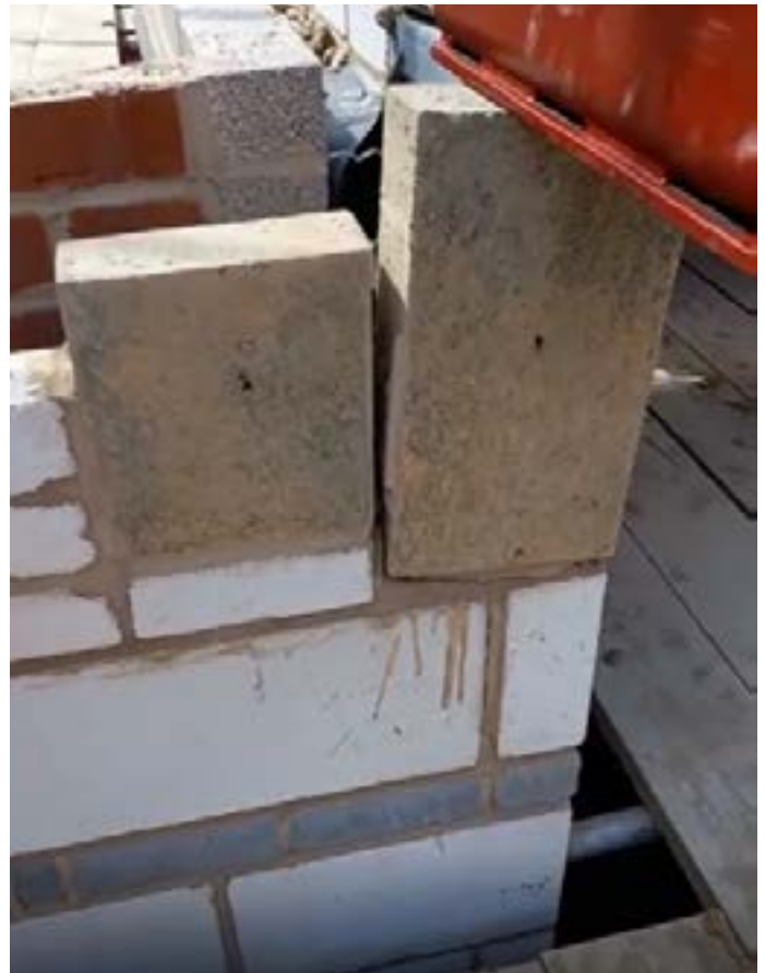
Figure 7 Example of unstable steel beam
