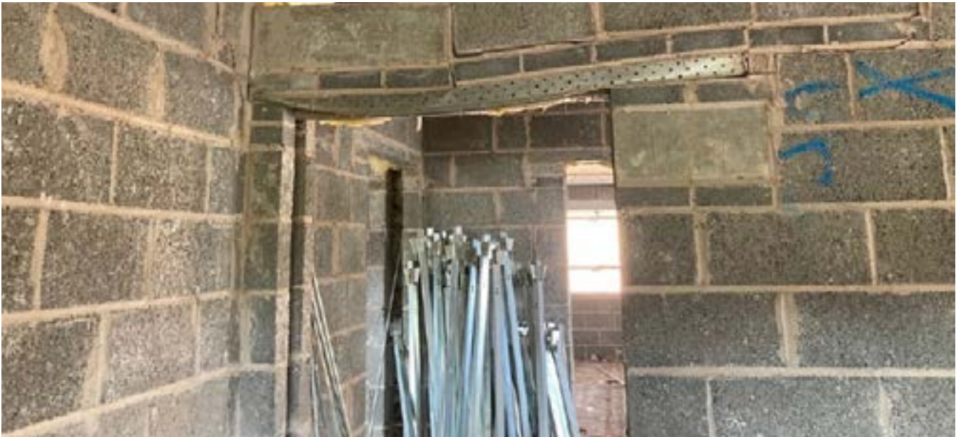
Figure 10 Failure of lintel
