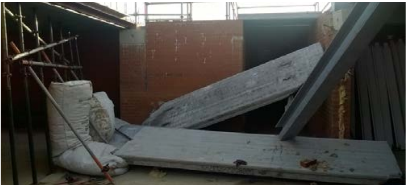
Figure 11 Failure of supporting steelwork due to inadequate propping detail
