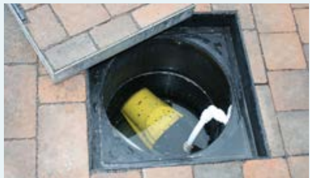
Around this home, rainwater runoff collected from all impermeable surfaces including roofs and paths, together with the 60m 2 permeable drive itself, passes into the tanked permeable pavement which contains a concealed sump. Here, a small pump is used to draw off the harvested water, in this case for outside uses, via a tap and hosepipe.
