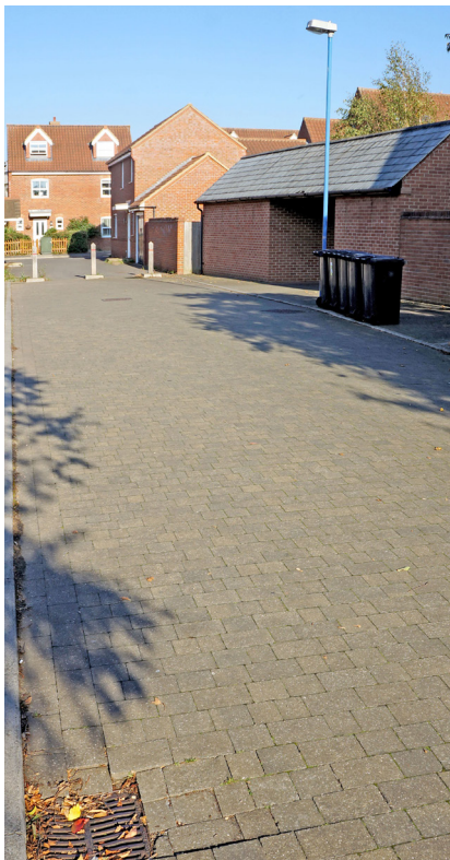
The impermeable block-paved courtyards offer negligible amenity value and no green space – a missed opportunity for SuDS.
